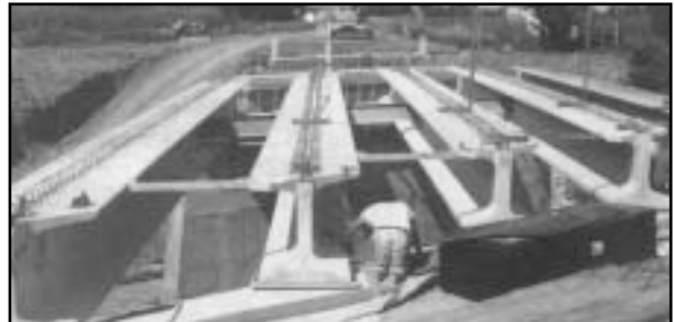
A bridge on Highway 8 in Salem, Neb., uses girders that were designed and fabricated in metric. A second metric girder bridge is in the works.
