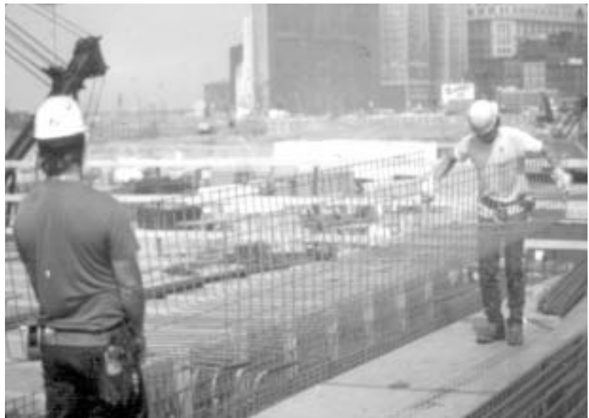
Bent cages of WWR for shear reinforcement in the poured, in-place concrete girders are easily handled by two workers.
