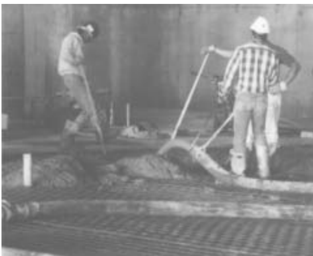
Workers ensure the proper WWR cover as they work with the pumped concrete.
