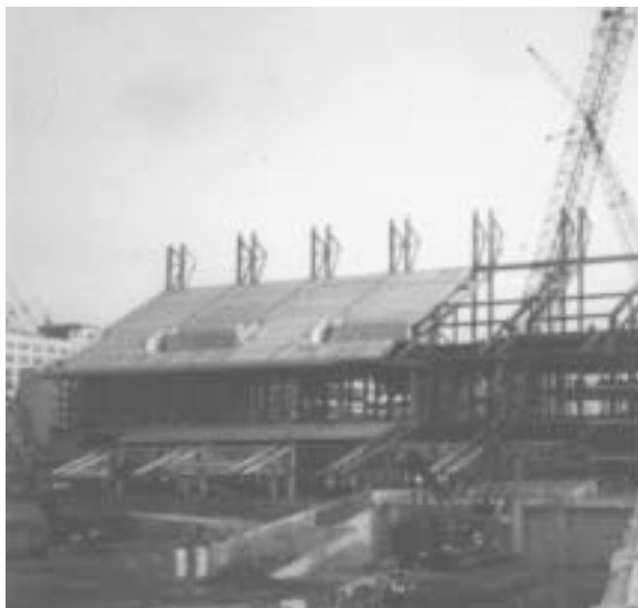
Precast concrete tiers for seating are reinforced with sheets of welded wire reinforcing.
